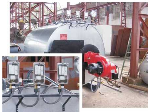
Picture shows 3x precision pressure switches MANOCOMB® model IP65 version 1K used as pressure monitor and pressure limiter respectively for boiler operation.
